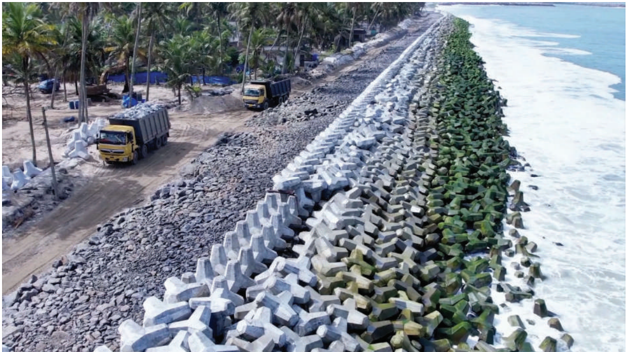
Fig 10.4 The seawall is already being scoured by the waves! Credit: ULCCS Ltd
