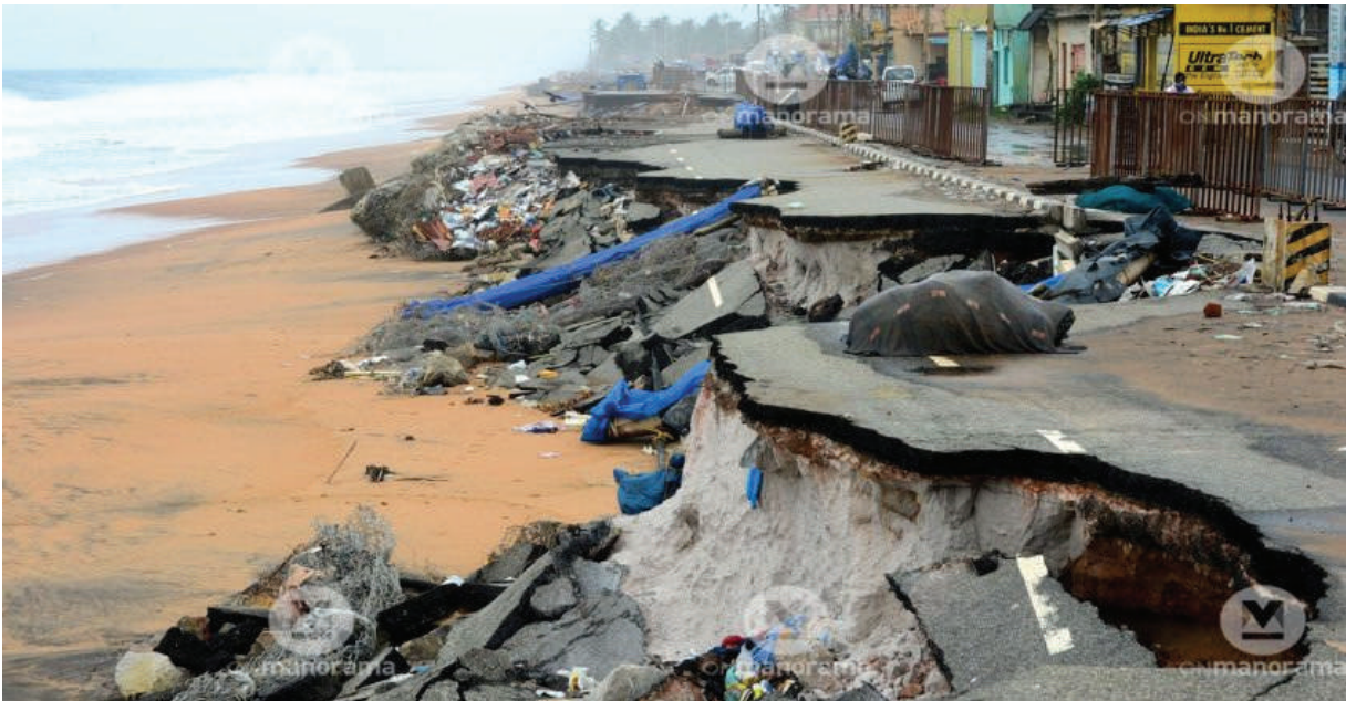
Fig 8.3: Shangumukham Beach Road to the Trivandrum International Airport destroyed by the waves. File photo: Manorama
