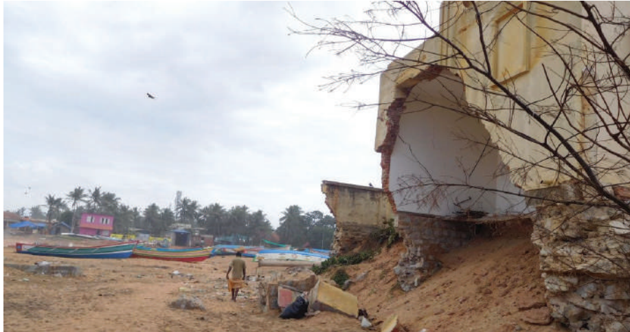
The National Centre of Earth Science Studies (NCESS) building in Kerala's Thiruvananthapuram district was damaged by sea erosion.
