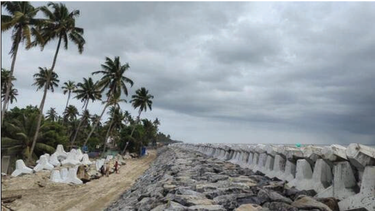
Fig 10.1: Seawalls of Chellam (2022): Perhaps a coastal engineering marvel, but an ugly eyesore and not a solution
