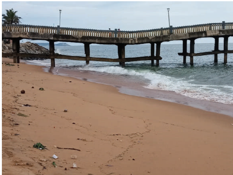
Fig. 5.16. Wide beach gradually got reduced as is seen in Nov 2022 and the Valiyathura pier itself got damaged and became unusable – fair weather beach totally disappeared south of pier while the width of fair-weather beach considerably reduced north of pier
