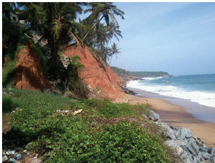
Fig. 5.5. Eroding cliffs south of Vizhinjam Fishing harbour almost at the VSL site (Credit: Neelima 2017)
